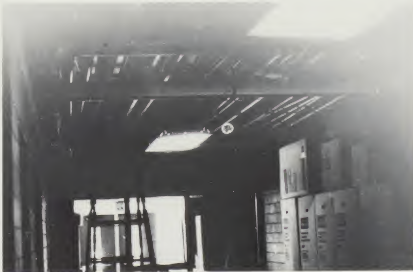
With the ceiling tiles out, it made walking through the halls seem like crawling through a cave.
